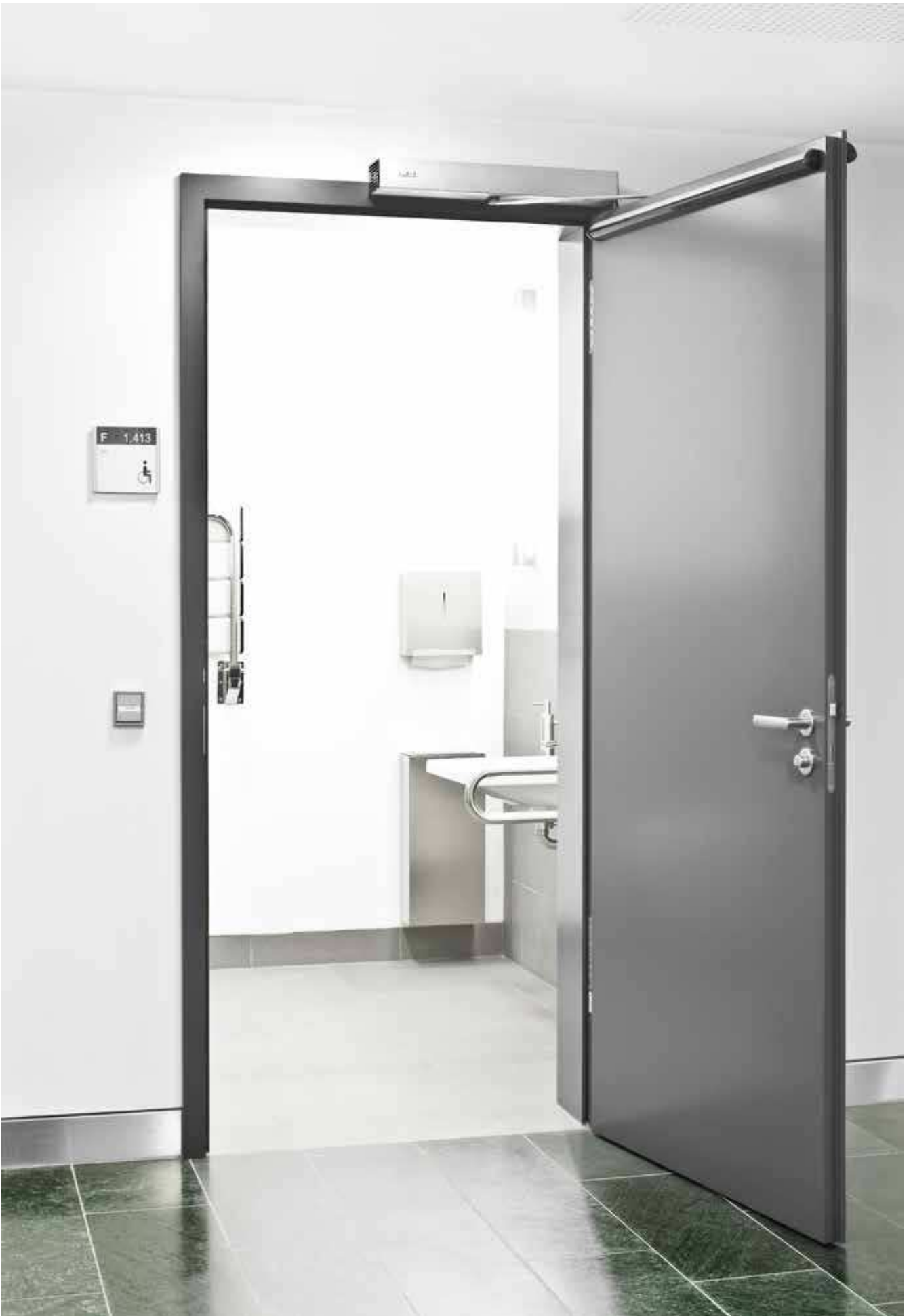
Slimdrive EMD-F swing door drive with GC 338 sensor strip, VGH Versicherungen Hanover (photo: Lothar Wels / GEZE GmbH)
